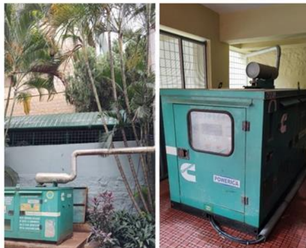
Figure 5-3: Diesel Generator (DG) set #1 and #2
