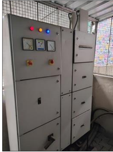
Figure 5-2: Electrical panel Room
