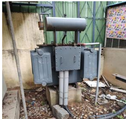
Figure 5-1: Transformer unit Installed in the campus
